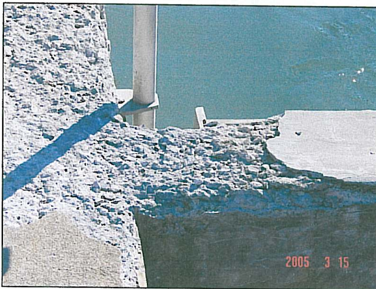
Concrete spalling at mixing basin
