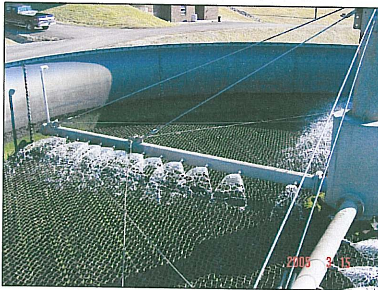
Town of Orange Sewer Plant Trickling Filter
